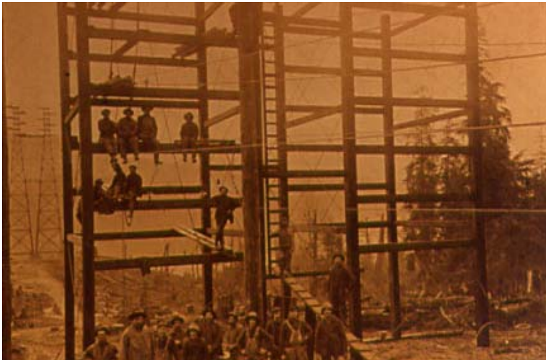
Hydroelectric transmission line construction from Buntzen power plant at Indian Arm to Greater Vancouver.
